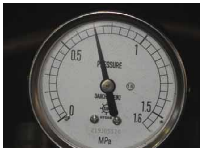
Test pressure 0.7 MPa. No pressure drop.
