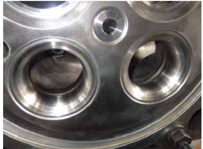
Exhaust valve seat no water leak.
