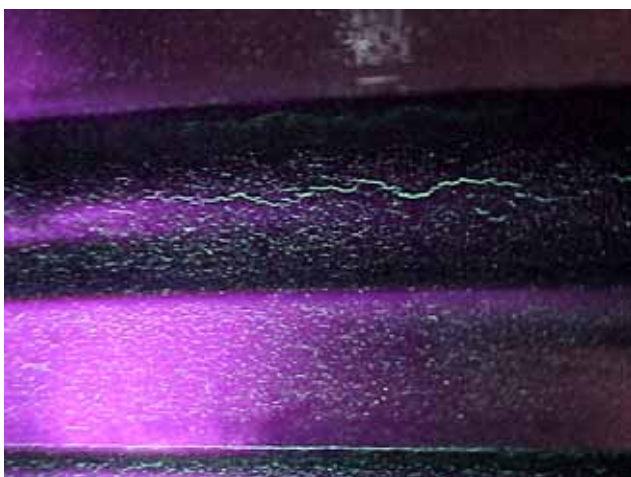
Example of crack: The crack occurred at under of the liner mounting surface. ライナー錨下クラック発生見本
